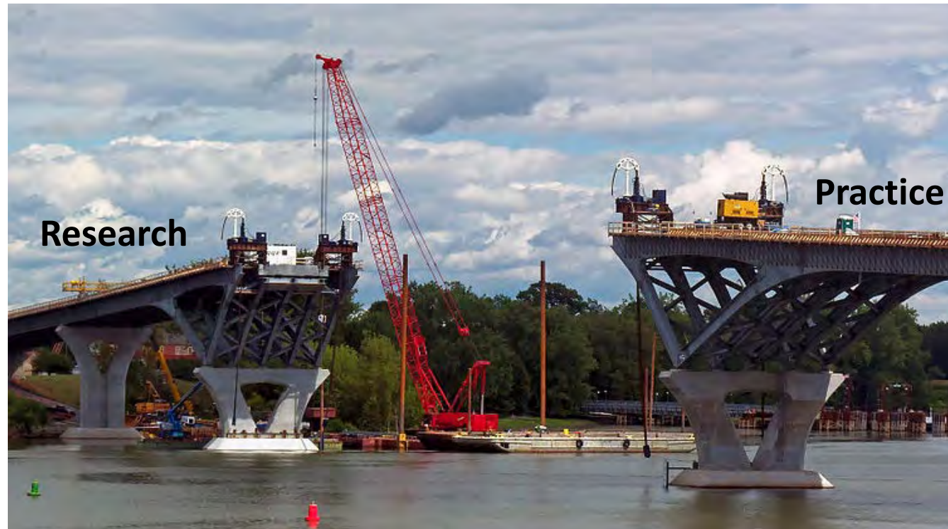
New Crown Point Bridge under construction between states of New York and Vermont, USA}} Author, Daniel Case |Date 2011-08-23, https://en.wikipedia.org/wiki/Crown_Point_Bridge
